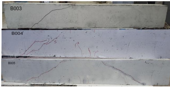
Figure 5. Crack pattern of group one ferroccement beams
