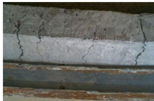
Figure 3: Cracks in concrete deck
