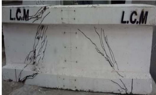
Fig. (2): Shear cracks pattern of L.C.M beam.
