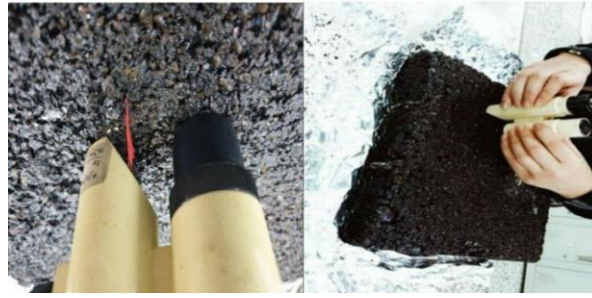
Figure 12. Measuring of cracks at asphalt layer.
